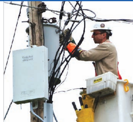
Installation of an ENGO unit on the secondary side of a service transformer.
